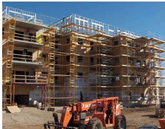
Bella Sera Our experience and reliability can reduce the time and expense of your new construction project.
